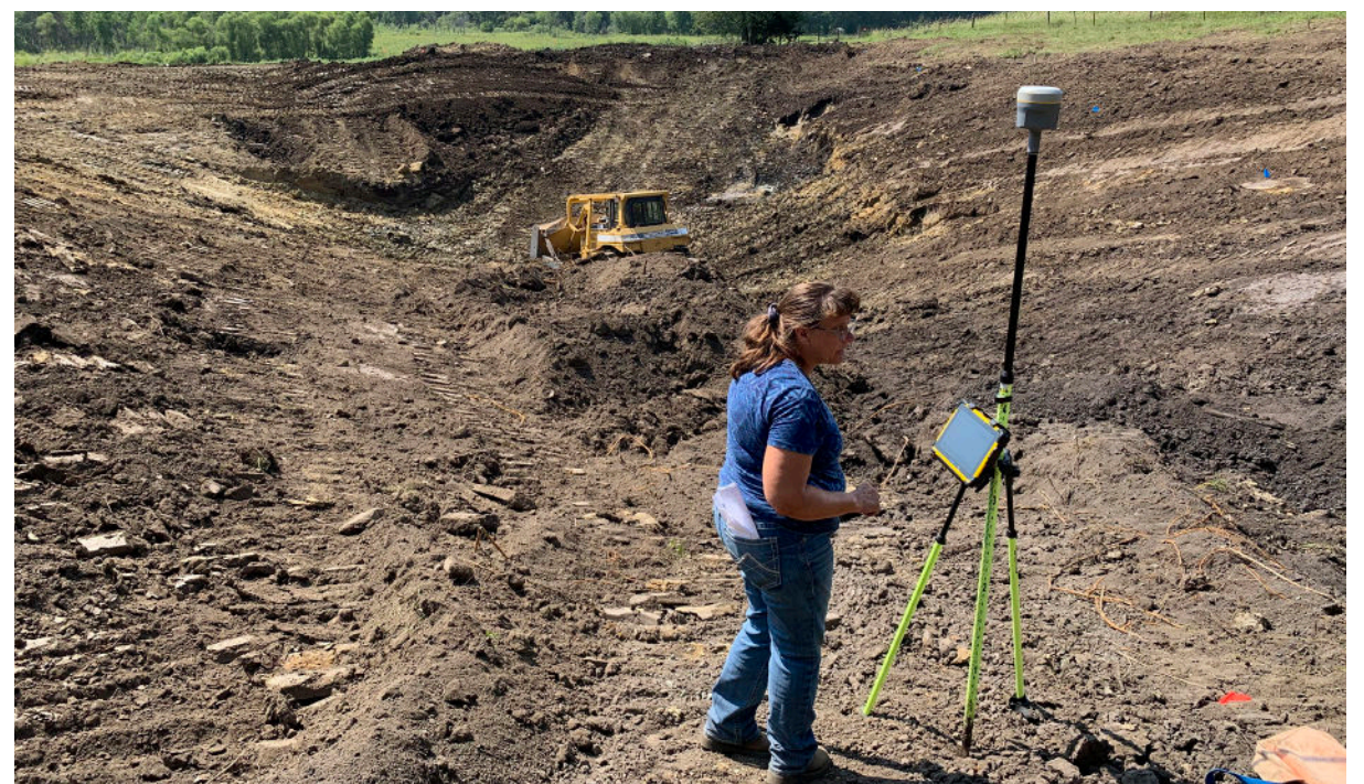
A livestock water pond under construction cost shared through the federal EQIP program.
